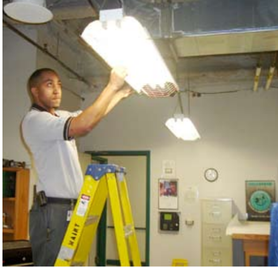
High-efficiency overhead lighting systems can reduce lighting energy use by up to 70 percent, while improving light quality.
